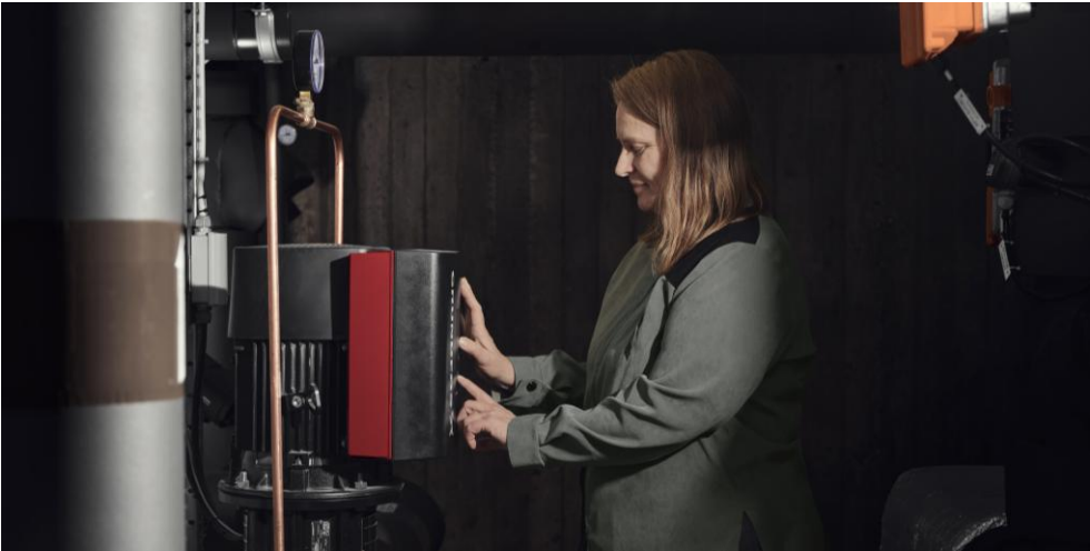
The geoenergy system at Pärönet 6, launched in May 2025, now supplies the property with heating and cooling and is expected to cut energy use by about 75%.
